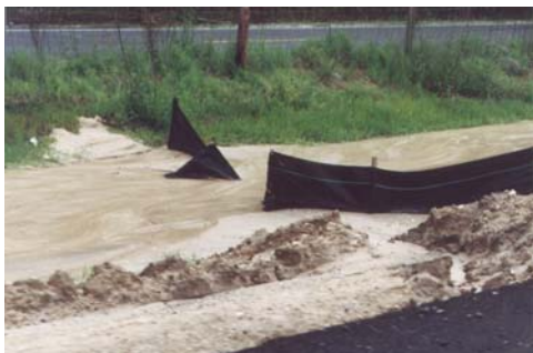
Figure 2. Failed silt fence check dam.
